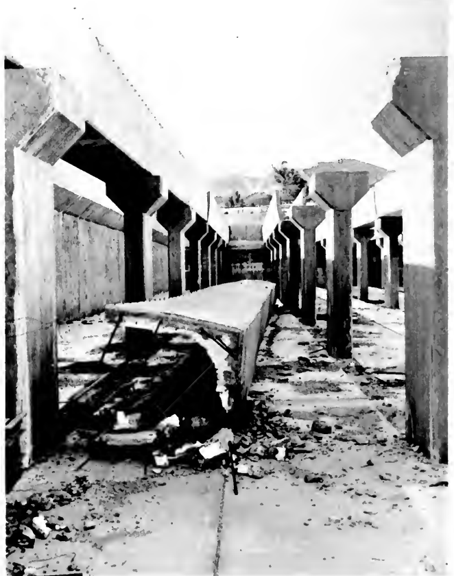
Photo 14. Joseph Jensen Filtration Plant. Launder columns and launders in west end of south settling basin. Launderers fell from atop columns. Metropolitan Water District photo.
